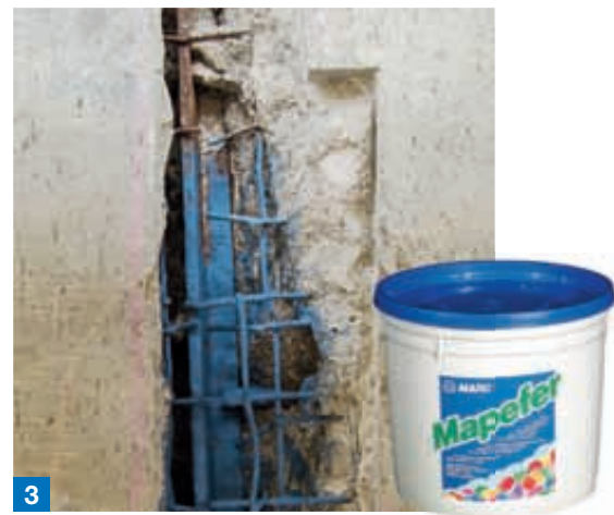
Photo 4. 2007-2008: repairing of certain sections of the Museum's circular outside facade using PLANITOP XS mortar.
