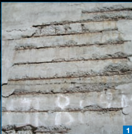
Photo 1. Close-up of the deteriorated concrete surface of one of the pillars on the viaduct before the restoration operation.
