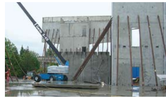
The Mapei manufacturing plant in Vancouver and the recent extension works on it.
