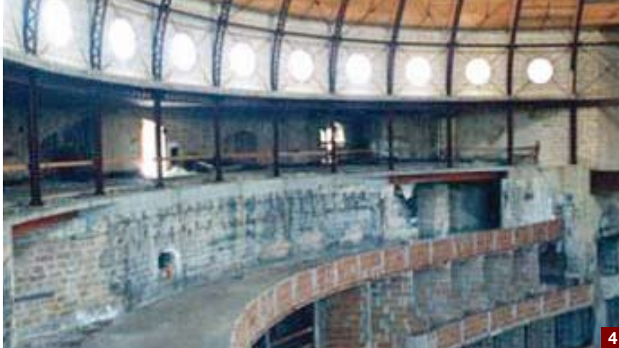
Photo 1. More than 6.000 m 2 of internal and external heated and normal screeds were laid using TOPCEM and TOPCEM PRONTO.
