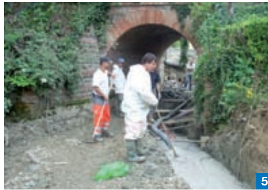
Photos 1, 2 and 3. Various phases of filling the trenches on the A75 motorway in France.
