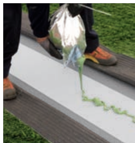
Application of ULTRABOND TURF PU 1K on the jointing tape via extrusion from its aluminum package
