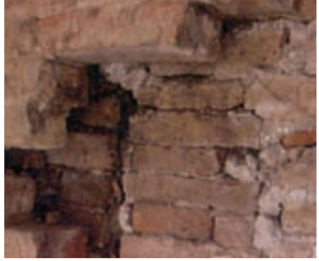
Photo 10. An image of the façade on Rio delle Torreselle before the restoration and maintenance work. The smaller photograph illustrates the level of deterioration of the masonry.
