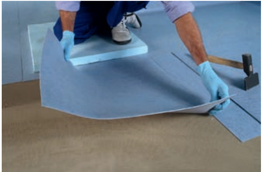
A good installation of PVC results from both good quality of the material and skillfull floor-layers.
