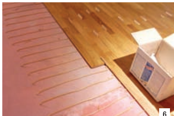
Photo 5. Before laying the parquet, the substrate was smoothed over with MAPESOL 3, a product available only on the French market. The equivalent product on the international market is known as PLANO 3. Photo 6. Following a request from the architect, a special template was used to form exactly the same gap between each parquet strip.
