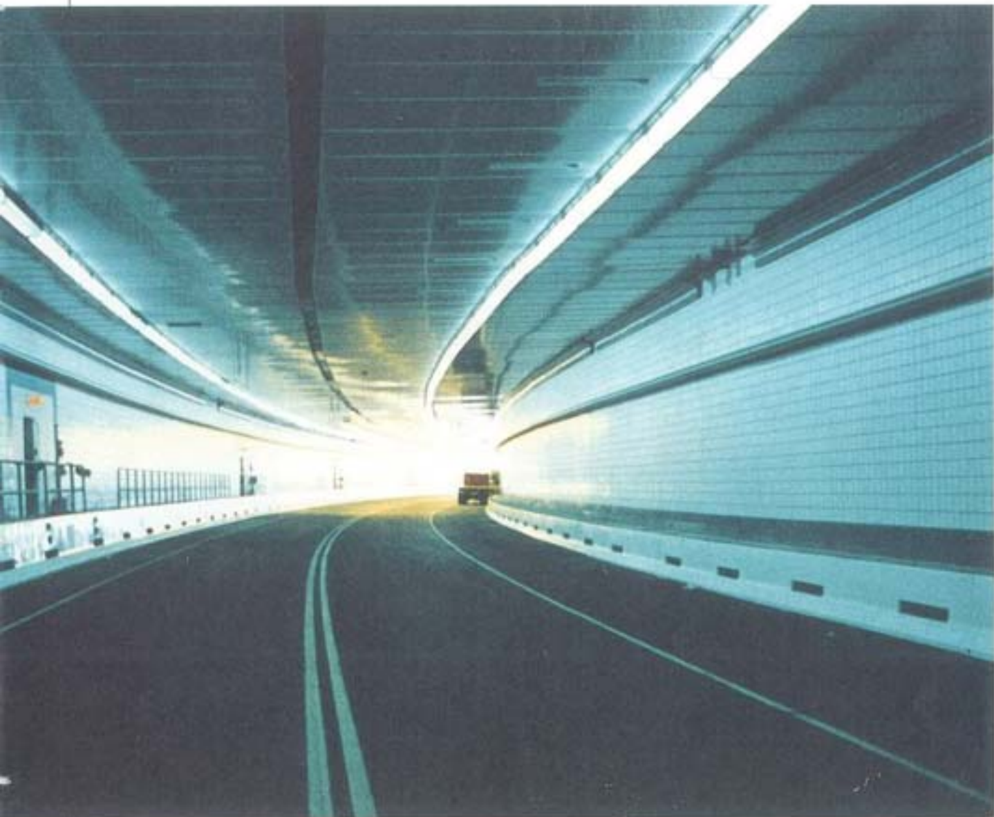
Photos 7 and 8 The "Central Artery" is ready to receive the thousands of vehicles that will pass...underwater!
