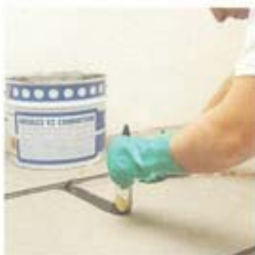
At left: installing copper strip with conductive polychloroprene adhesive At right, installing conductive pvc with conductive adhesive in water dispersion
