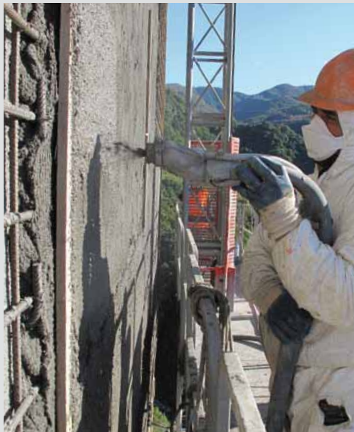
ABOVE. Applying by spray MAPELASTIC GUARD two-component, elastic cementitious mortar for protecting large concrete structures subjected to high stress. The product complies with the principles of EN 1504-9 and the minimum requirements of EN 1504-2 coating (C) according to principles MC and IR for protecting concrete.
