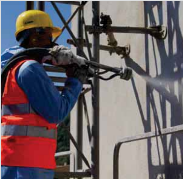
ABOVE. Applying by spray MAPEGROUT EASY FLOW one-component, fibre-reinforced, compensated-shrinkage, sulphate-resistant thixotropic mortar, particularly suitable for repairing concrete structures with a rendering machine. The mortar meets the minimum requirements of EN 1504-3 for class R4 structural mortars.
