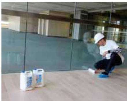
ABOVE. Wooden floors were bonded with LIGNOBOND adhesive and varnished with ULTRACOAT HIGH TRAFFIC to provide more resistance to foot traffic.
