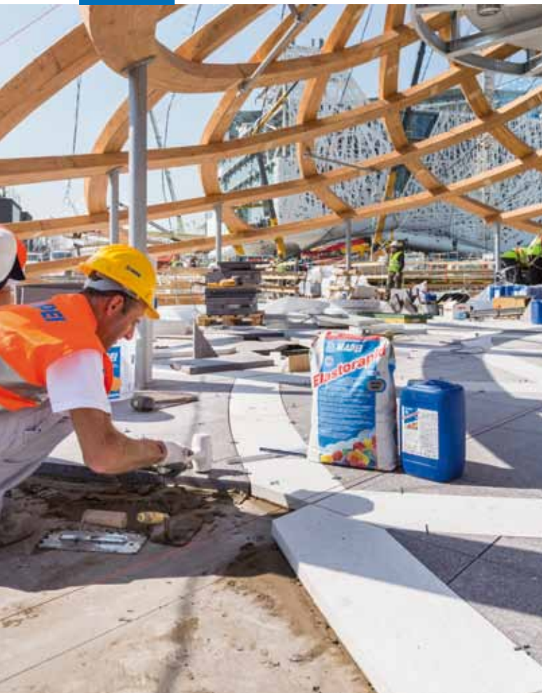
ABOVE. Mapei supplied the cementitious adhesive ELASTORAPID to lay the stone coverings at the base of the Tree. ULTRACOLOR PLUS was used to grout the joints.
