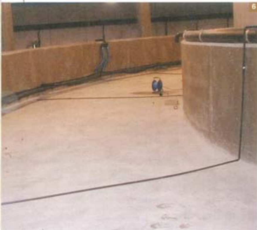
4. Fixing of the HDPE pipes into the wall of the main tank
