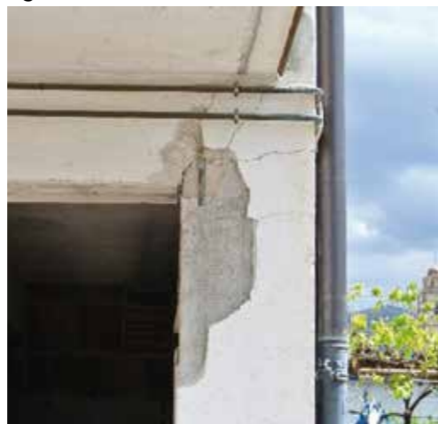
Fig. 1. Shear failure of beam-column joints following seismic activity (a), (b).
