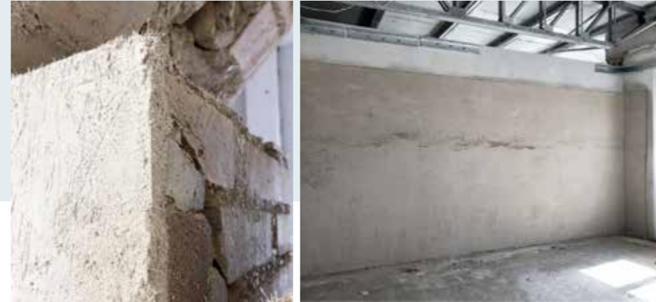
Close-up of the product applied (left) and the masonry panel after completing the strengthening work (right).
